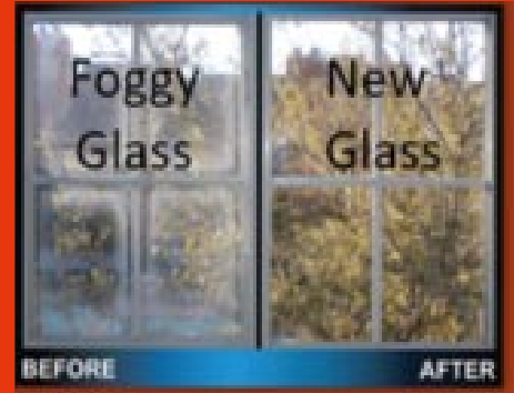
Foggy Glass Replacement
